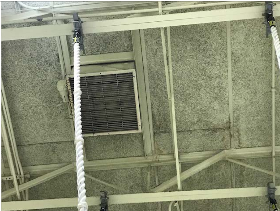
Photo 8: Physical Education Room – Air supply grills on ceiling contain excessive levels of dust.
