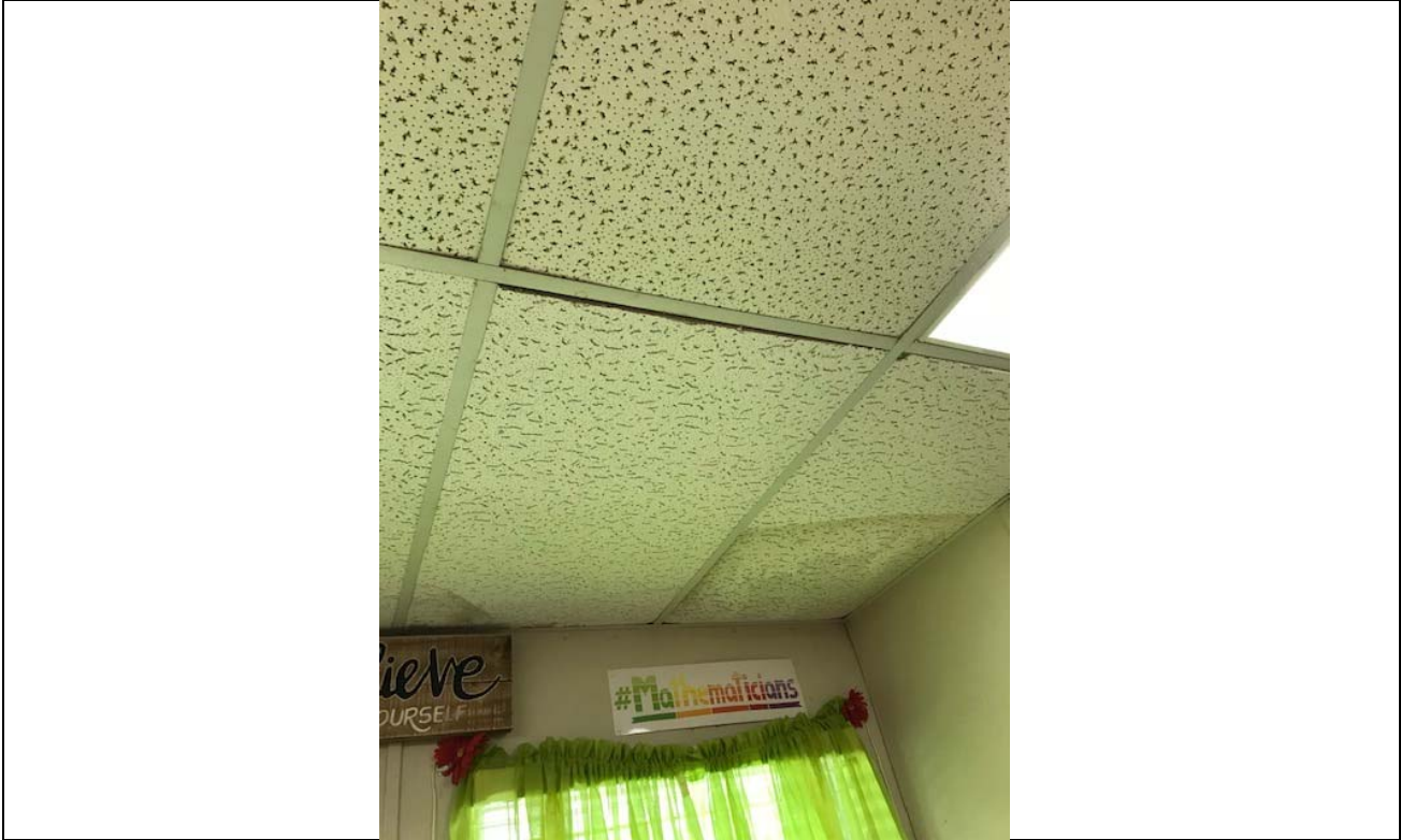
Photo 11: Classroom B2 – Water-stained ceiling tiles.
