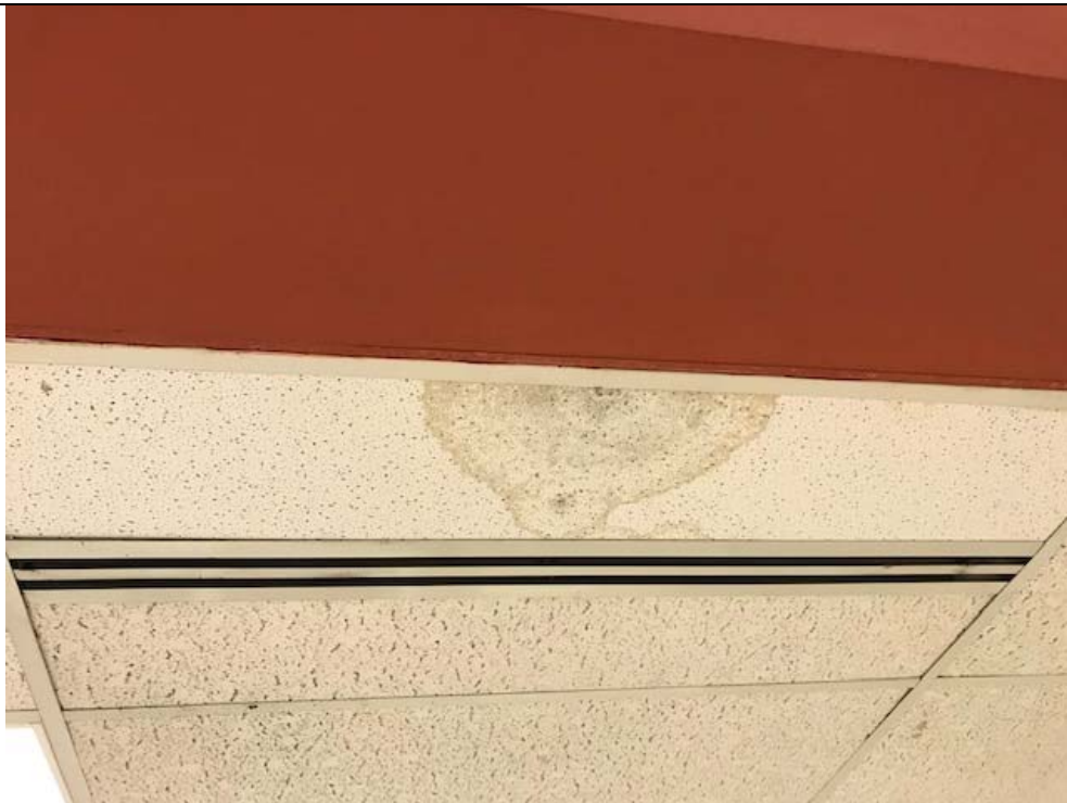
Photo 6: Library – Water-stained ceiling tiles.
