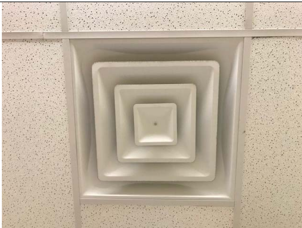
Photo 4: Classroom 205 – Ceiling-mounted Air Supply Grills clean.
