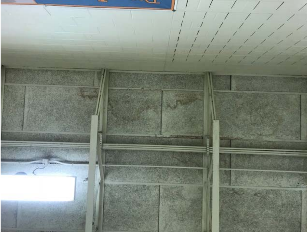
Photo 9: Physical Education Room – Water-stained ceiling tiles.
