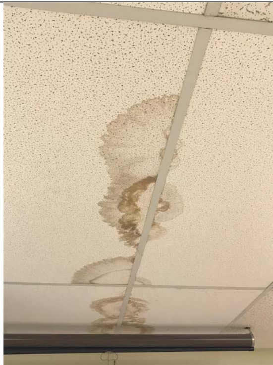
Photo 10: Classroom B2 – Water-stained ceiling tiles.
