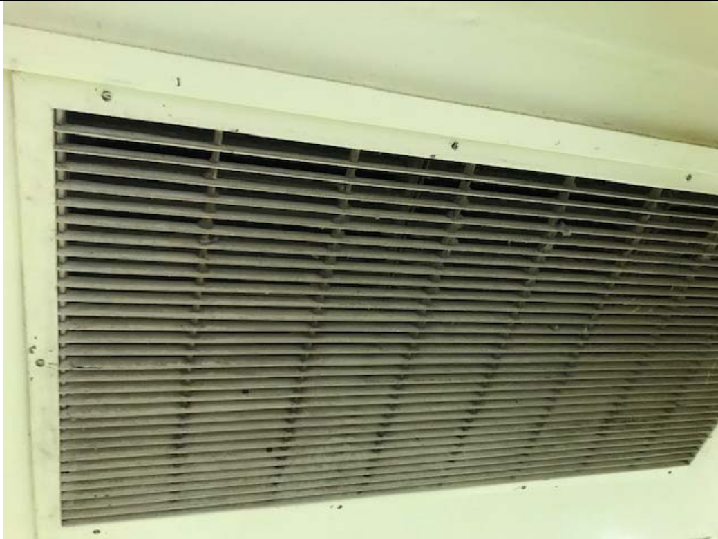
Photo 7: Physical Education Room – Air supply grills on wall contain excessive levels of dust.
