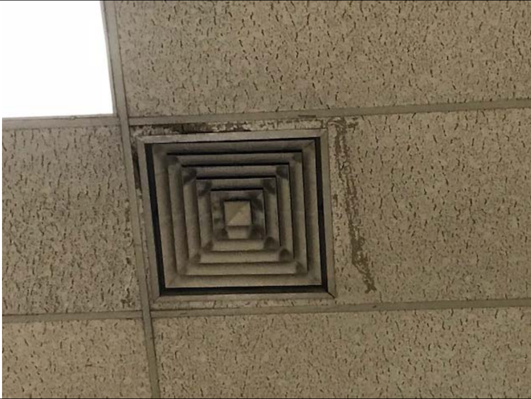
Photo 1: Cafeteria – Return air grills contain excessive levels of dust.
