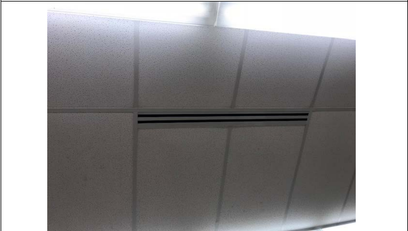
Photo 12: Classroom 302 – Clean air supply grills on ceiling.
