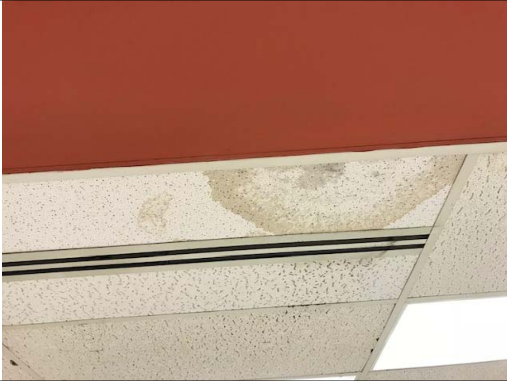
Photo 5: Library – Water-stained ceiling tiles.
