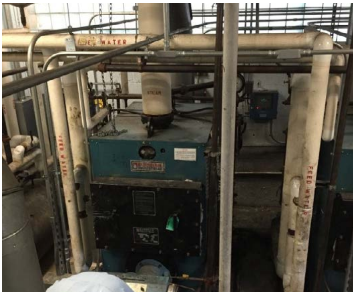
Orme Building: Main Mechanical Room
