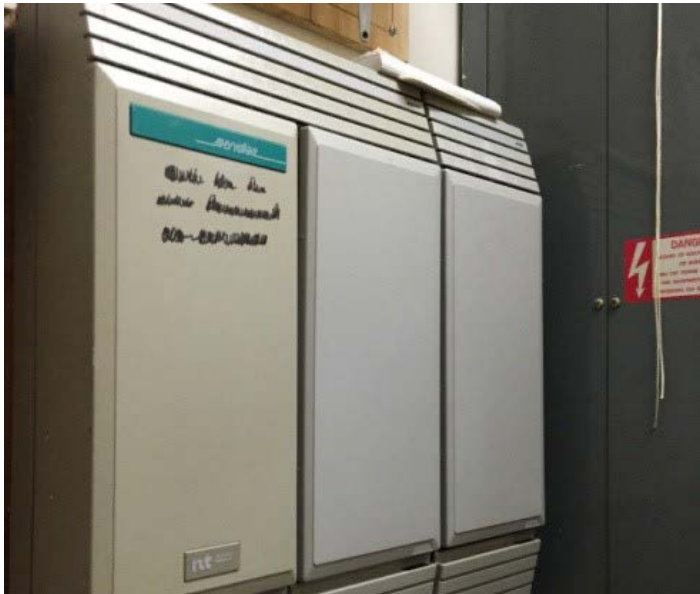
Admin: Tel/Data Components in Utility Room
