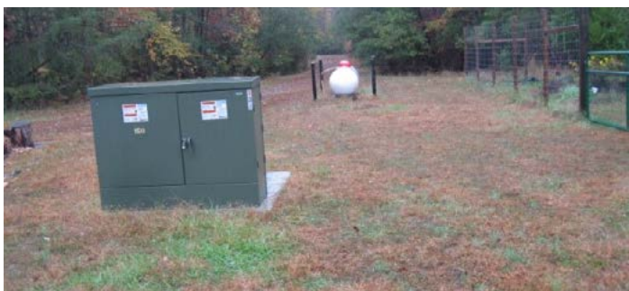
Admin: Existing Pad Mounted Transformer
