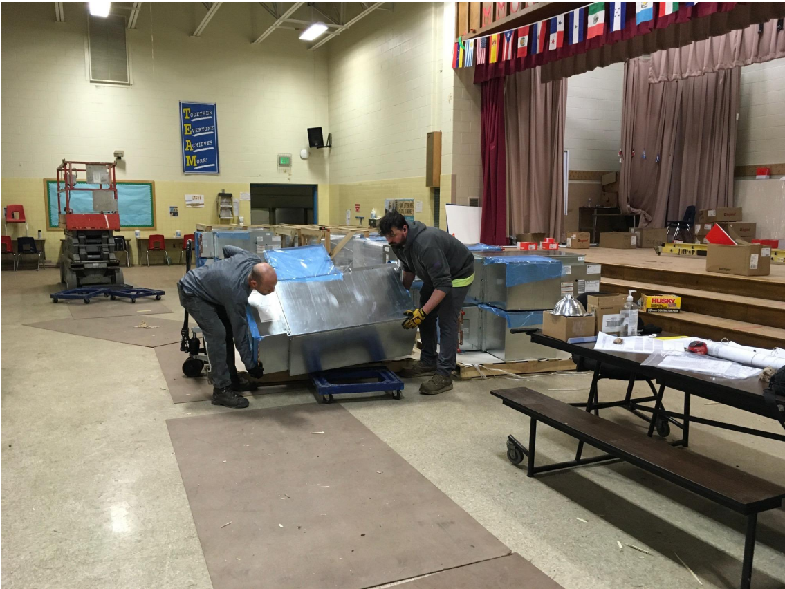
Delivered VAV currently stored in cafeteria, relocating to different rooms for installation
