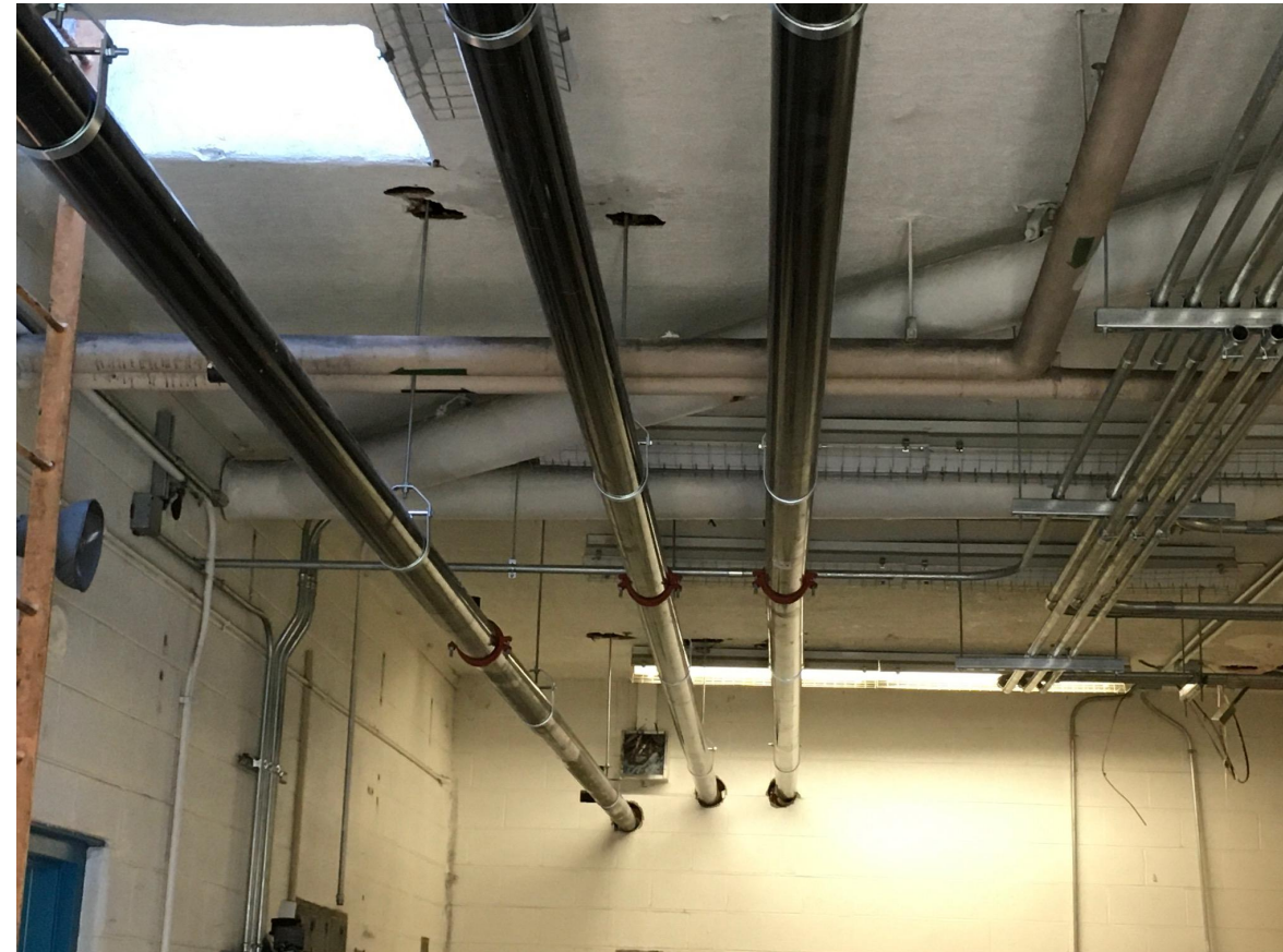
Newly installed sprinkler pipes connecting from mechanical room to the rest of the building
