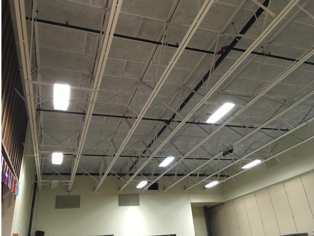
Newly installed sprinkler pipes and heads above the Cafeteria
