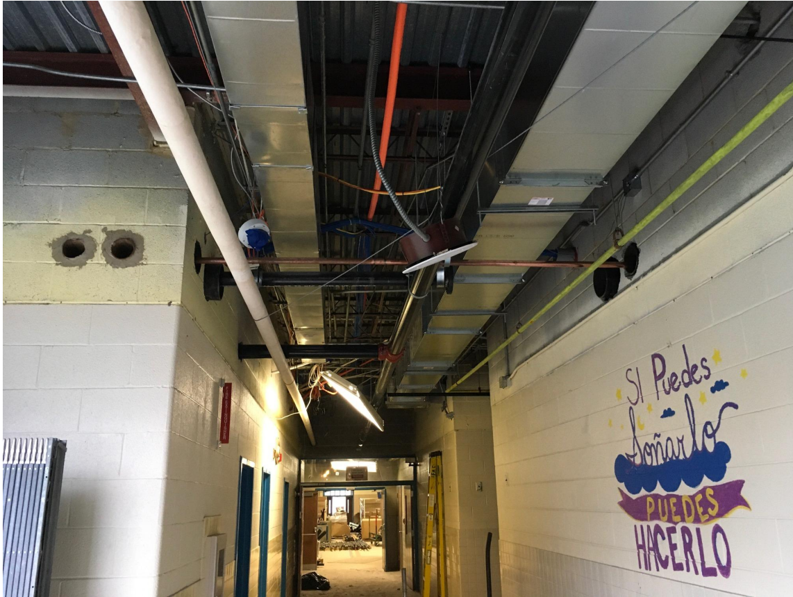
Newly installed ducts at corridor
